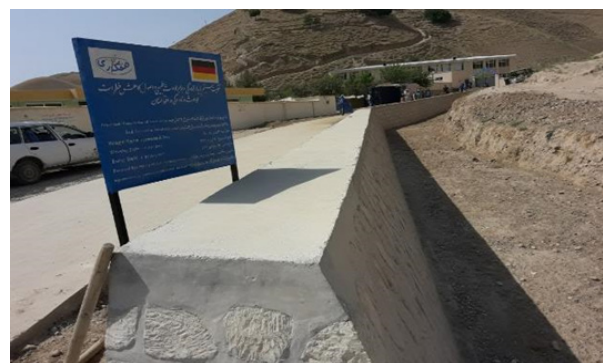
“ Picture shows the completion of the jamshidi high school protection wall project pashton kot district of Faryab province ”
